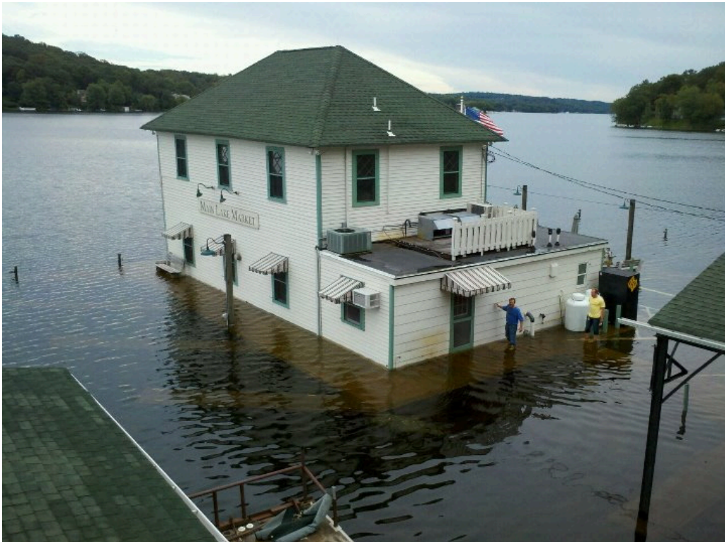
Main Lake Market during the flood of 2000. Photo courtesy of the Lake Hopatcong Historical Museum.
